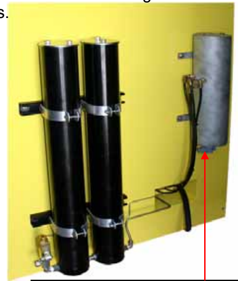
Condensate Drain Container. Check & Drain Weekly.
