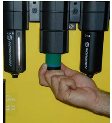
Changing LP Filtration Element
