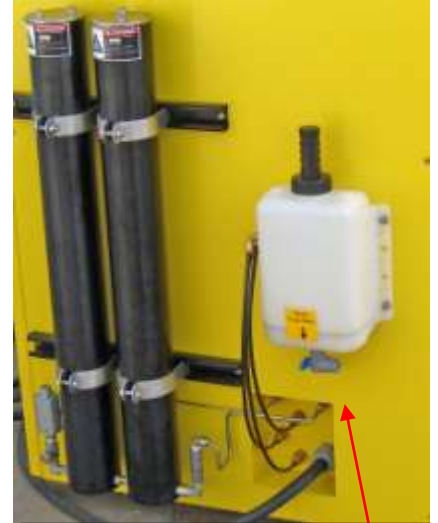
Condensate Drain Container. Check & Drain Daily.
